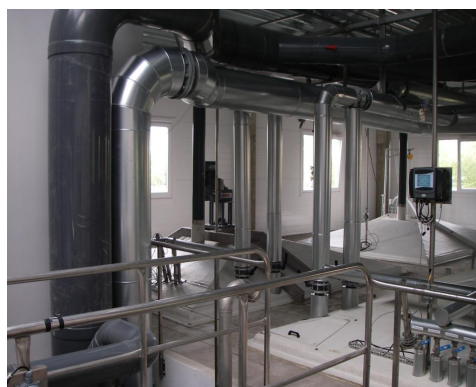
Covered MBBR reactors.
